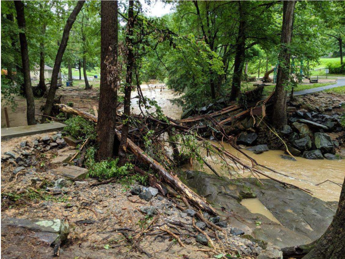
Figure 3: Damage in Glencarlyn Park, along Four Mile Run (photo courtesy Amanda Lowenberger)
