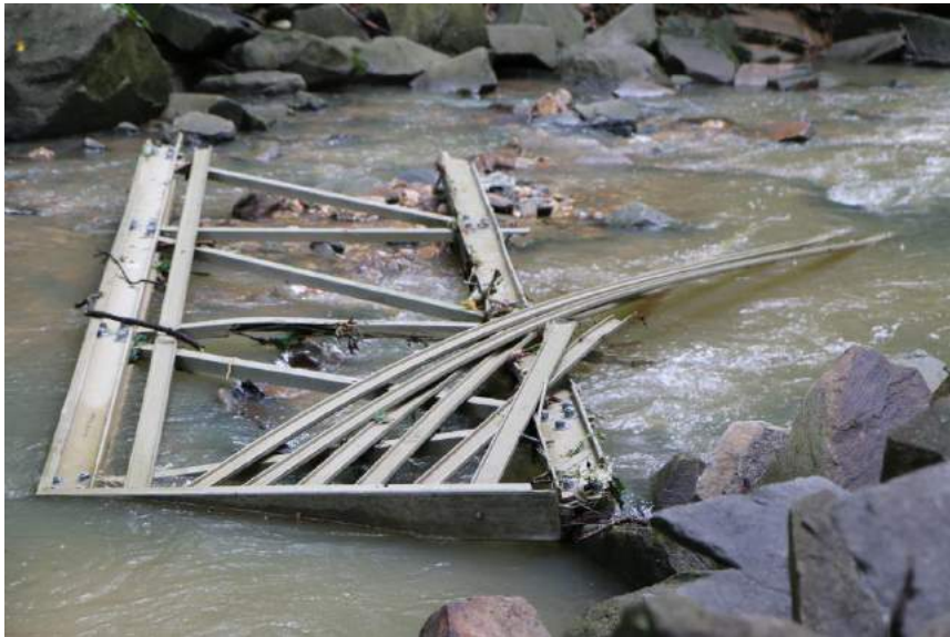
Figure 2: Pedestrian bridge washed away along Lubber Run (photo by Ashley Hopko)
